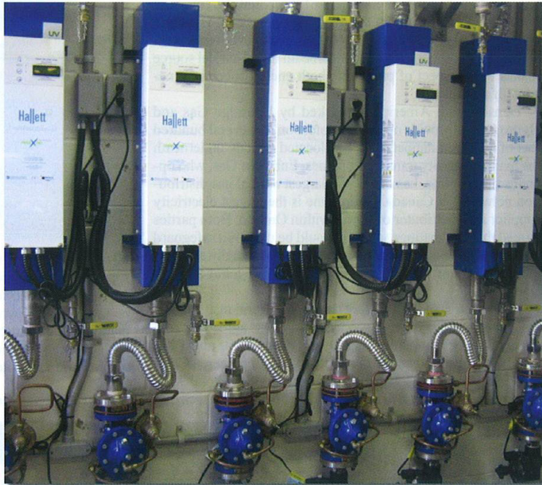
Hallett 30 UV units at Sunderland Water Supply System.
