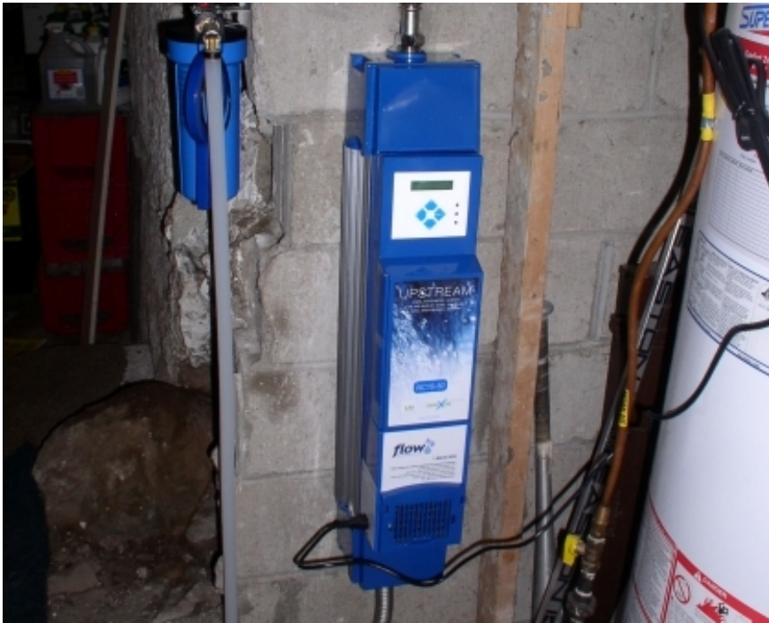
A Flow Water installation - Upstream 10-75 (10 gpm/75% UV)
