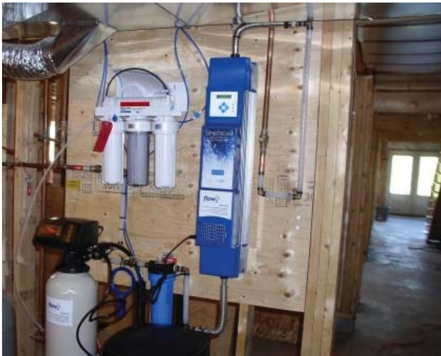
A Flow Water installation - Upstream 10-50 (10 gpm/50% UV)
