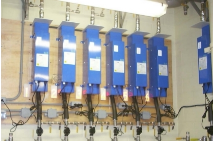
Initial installation in Baltimore, Ontario: 6 Hallett 30s in parallel, plus 1 for redundancy
